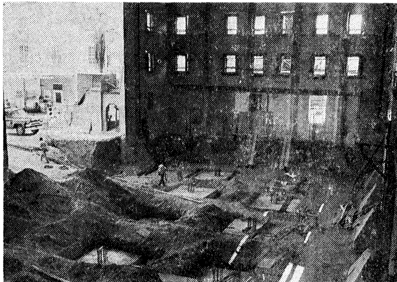
Construction is under way as a $1.1 million grant from the Sloan Foundation transforms the old High Voltage lab into a new Mathematics-Physics building.
