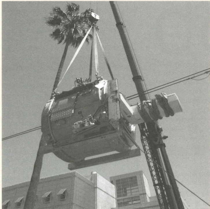
The Broad Center for the Biological Sciences received a load of equipment, including the first of three magnets for its MRI (magnetic resonance imaging) center, on Tuesday, April 8. In order to easily access the basement, where the center is located, the sidewalk south of the building was opened like a hatch. The second magnet is scheduled to be installed in September 2004.
