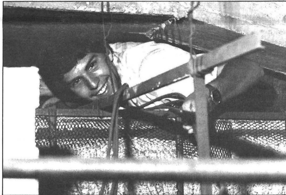
Junior Greg Gallagher explores a little-known nook of Ricketts House as he lays cable that will connect the house with the campus computer network, ETHERNET. Over the summer, the network was expanded to include the student houses, with students installing the cable and outlets.
