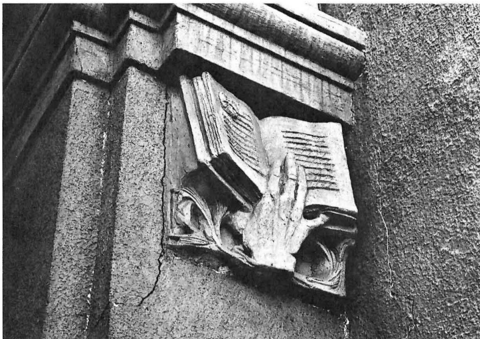
Throop Hall received new cracks, but no structural damage.
