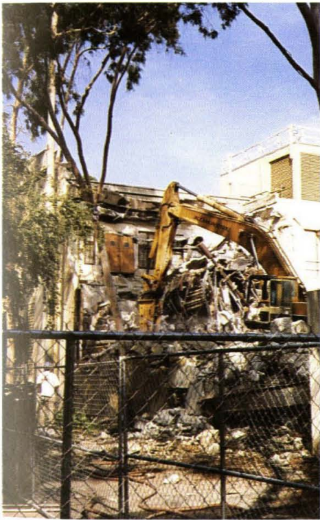
Above: Bulldozers destroy the old Chemical Engineering Laboratories, which once functioned as a cool entrance to the tunnels.
