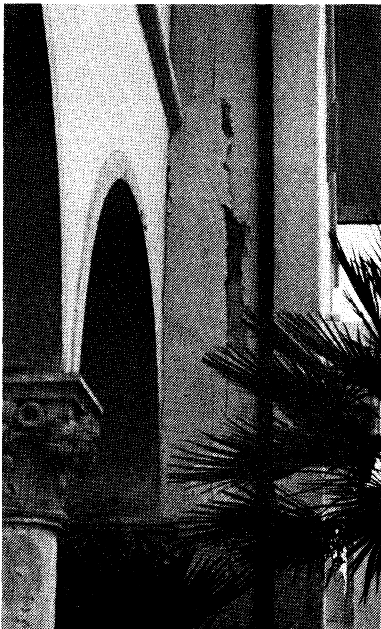
A considerable amount of plaster fell from the newly-renovated walls of Fleming and Ricketts Houses. No structural damage is suspected.
